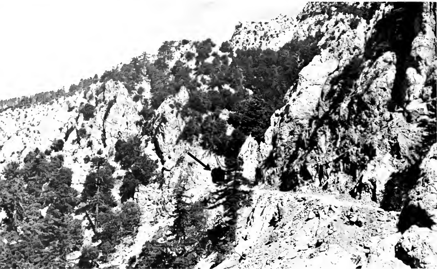
Arrow points to tunnel No. 1 under construction through ridge of Mt. Williamson on Angeles Crest Highway in San Gabriel Mountains
